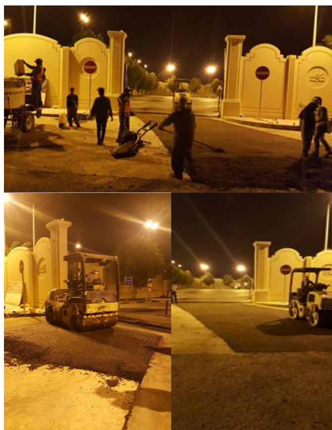
Figure 14. Mixing, placement, and compaction of the G5 ® -stabilized RAP mixture at Al Wakar water station in Doha.
